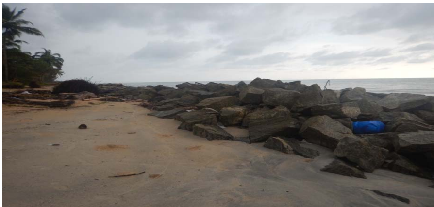
Fig. 4.13 Partially destroyed seawall and uprooted trees due to beach erosion
