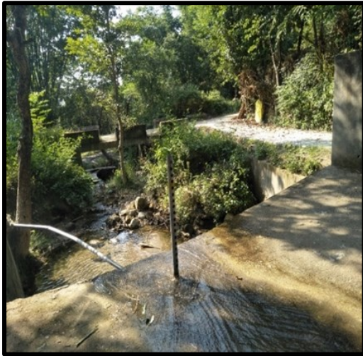
Figure 41. Sediment collection pipe
