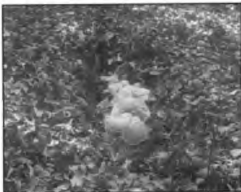
Plate 11. Neglected rain pit in Elanad
