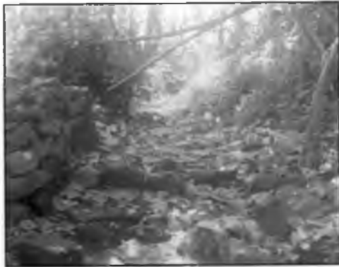
Plate 13. Neglected loose boulder check dam in Elanad
