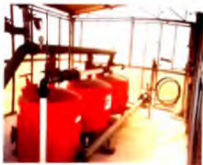
Primary Filtration Station and Water Supply System
