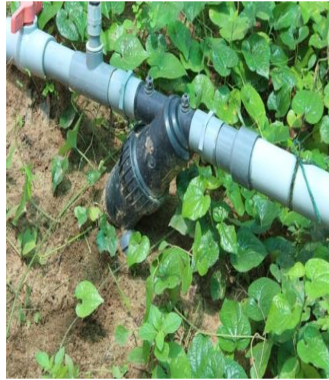
B) Filtration unit
