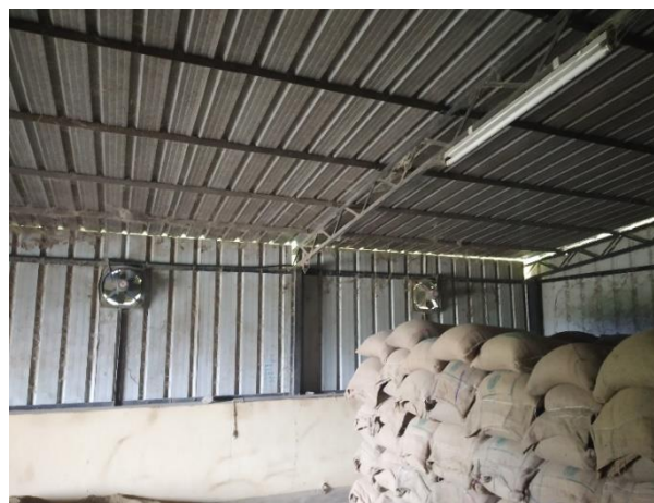
SC1 (Asbestos + forced ventilation)
