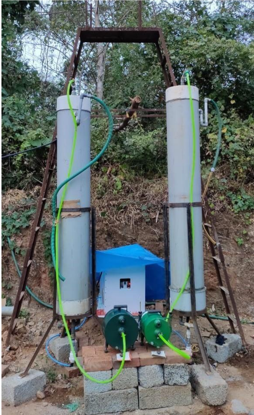
Fig. 3.7 Pilot scale UAHBR installed at rubber latex processing unit
