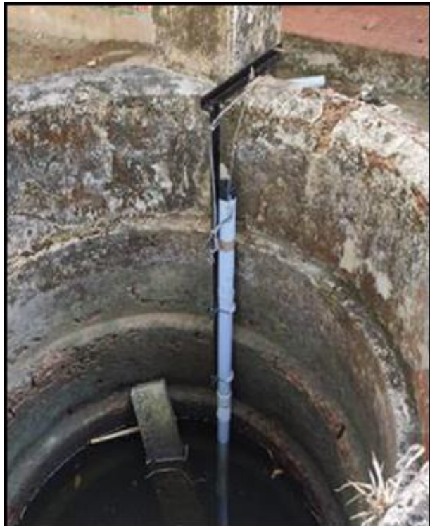
Fig. 3.22. EMCON Automatic Water Level Sensor Installed in the Open Well
