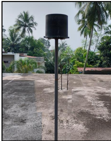
Fig. 3.4. Tipping Bucket Rain Gauge Installed in the Study Area
