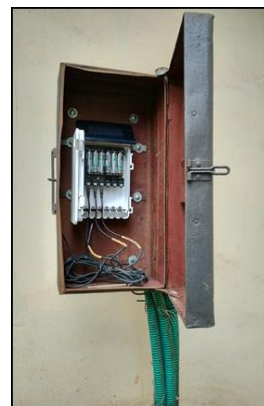
Fig. 3.16. ZL6 Data Logger Installed in the Study Area
