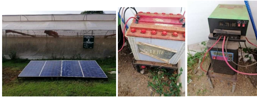
Plate 3.10 Solar power supply
