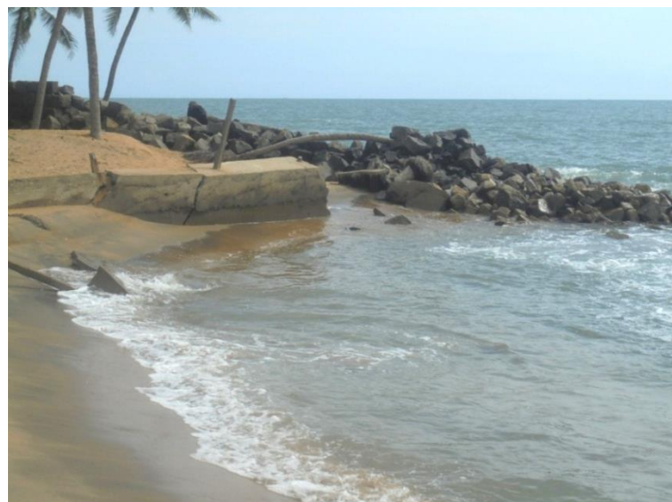
Plate 4.6 Erosion at the end of the structure
