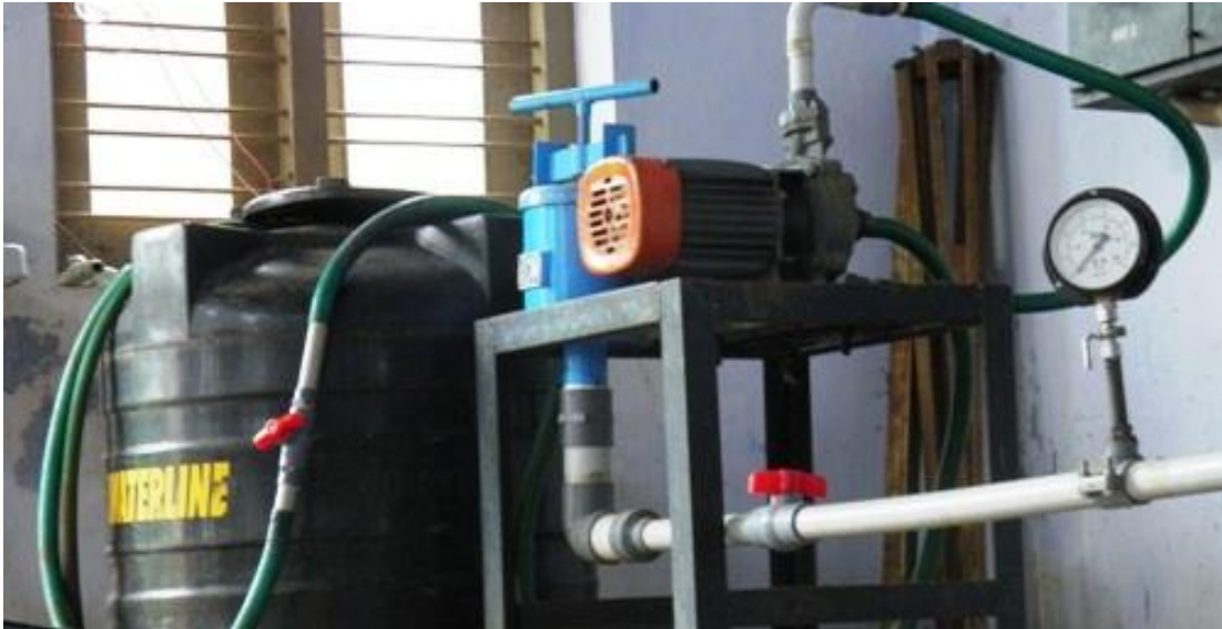
Plate 3. 4 Test set up of micro sprinkler: pump, pipe and control valves
