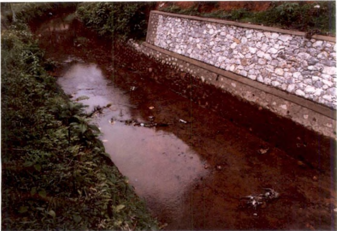
Plate 4.3 Improper maintenance of canal
