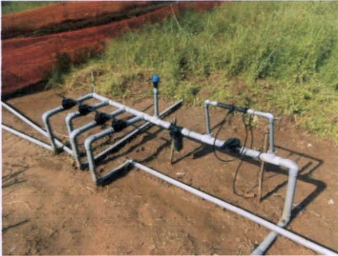
Plate 3.7 Control head of drip irrigation system
