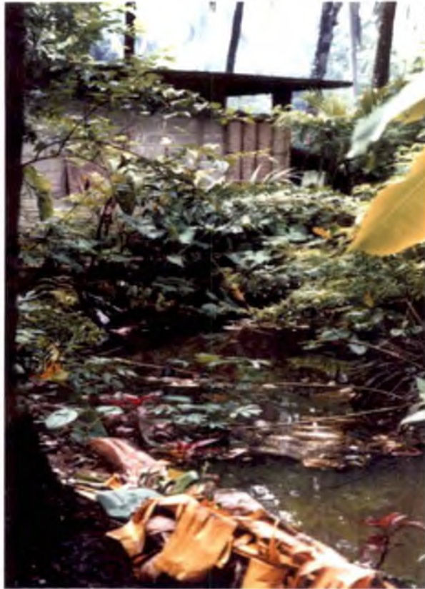
Plate no. 6. Poor drainage facility observed in the study area
