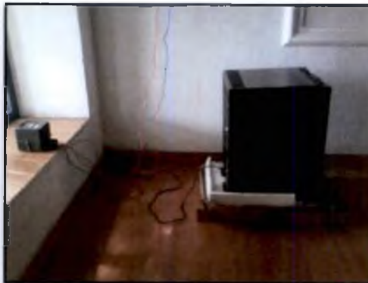
Plate 3.10 VARS with energy meter
