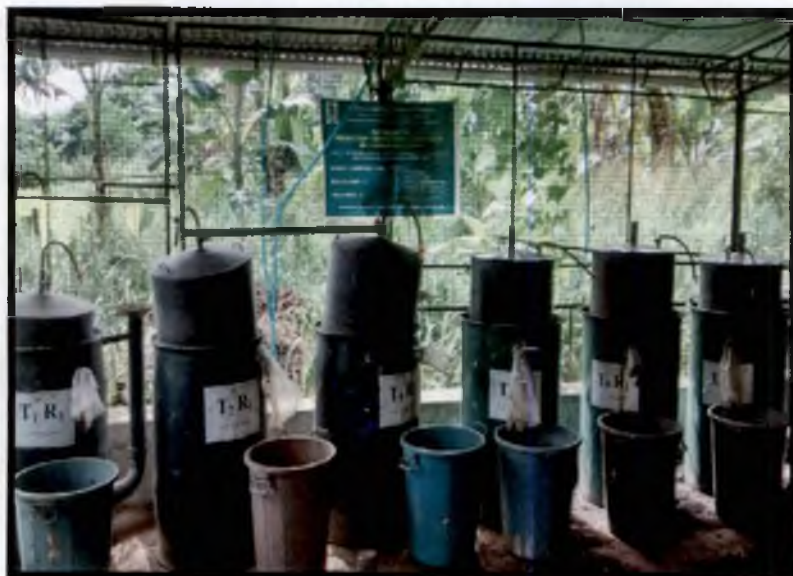
Plate 2. Anaerobic digestion of substrate in biogas plants
