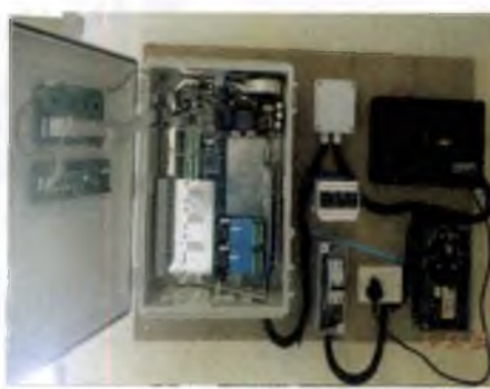
Plate 3.3 Open view of MCU
