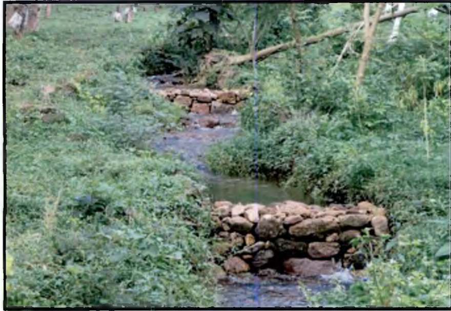
Plate 4. Loose boulder check dam
