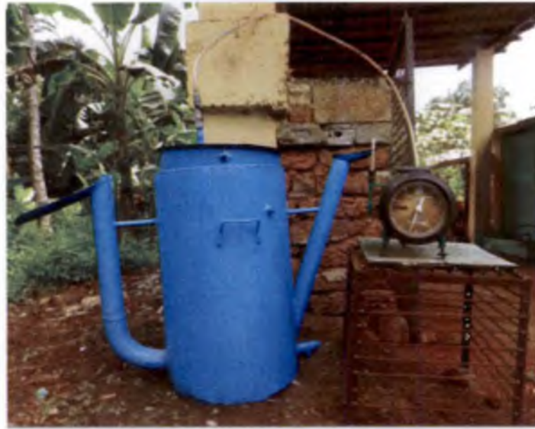
Plate 3.5 Floating gas holder digester with wet gas flow meter installed at oil mill
