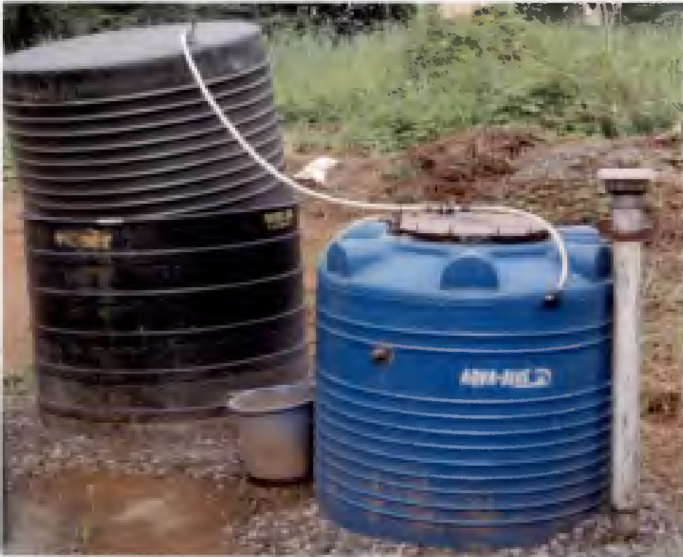
Figure 14. KAU split biogas plant
