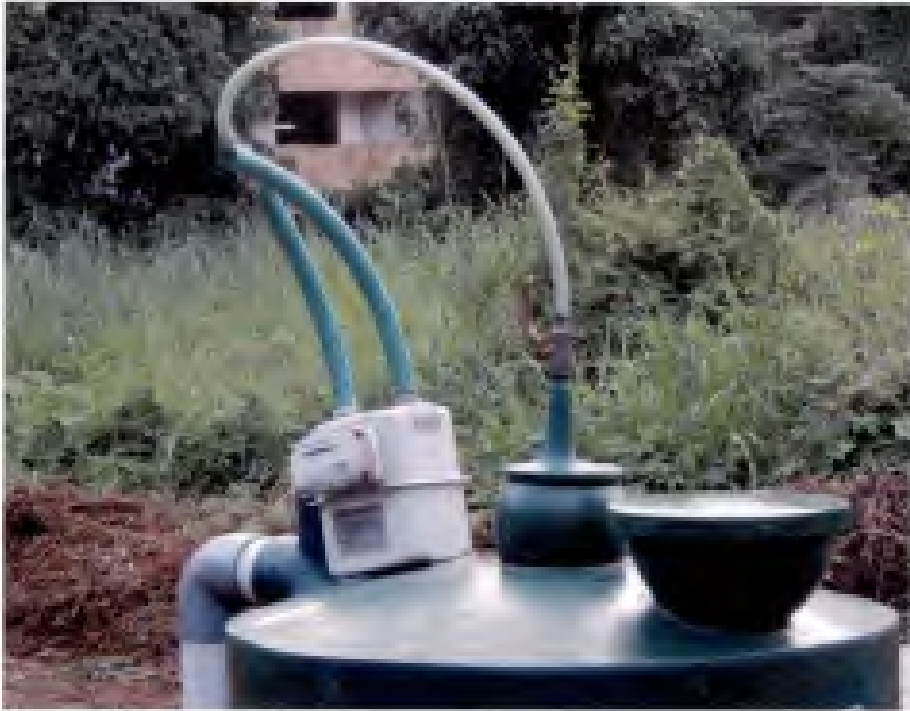
Figure 17. Biogas flow meter
