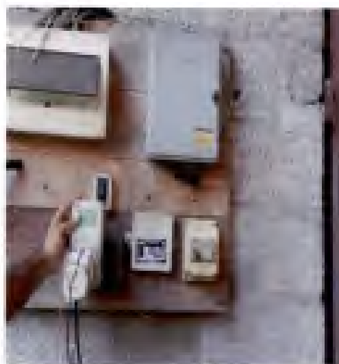
Figure 4. Single phase power meter
