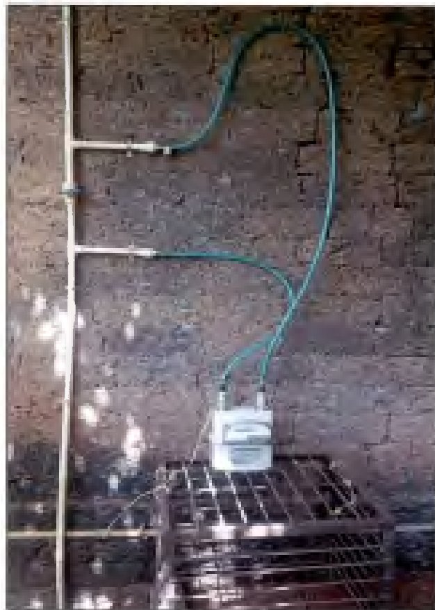
Figure 7. Biogas flow meter
