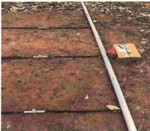
Plate 3.200 Automation Components setup
