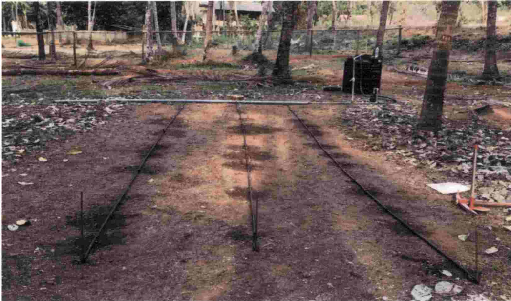
Plate 3.19 Setup for Automated Pulse Drip Irrigation System
