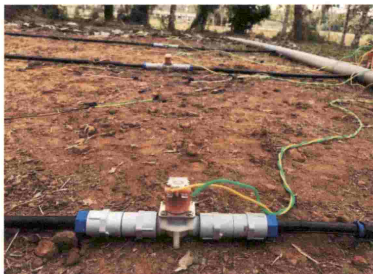
Plate 3.23 Solenoid Valves controlled by corresponding moisture sensors
