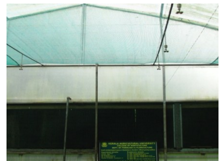
Inside view of fan and pad system
