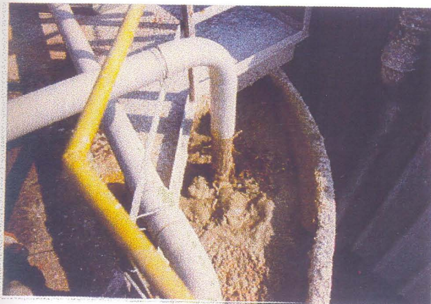
Plate 2 Thickner slurry pump site
