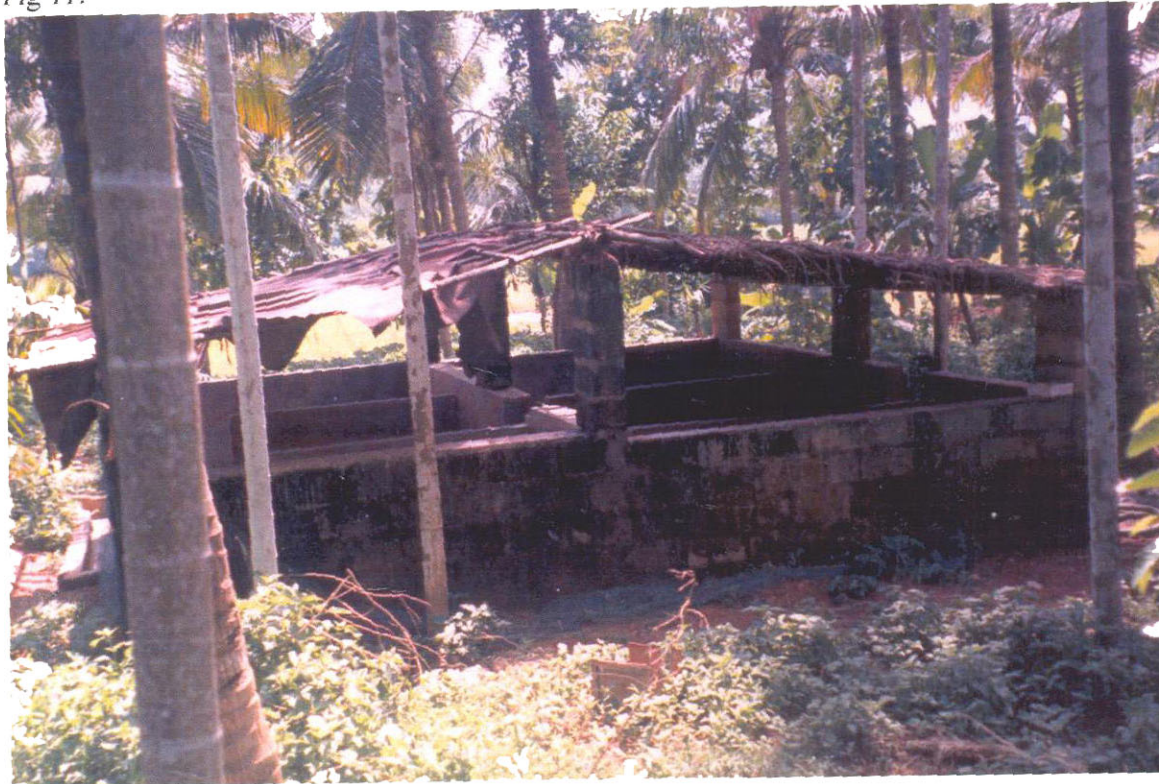
Fig 10 & 11 Pig house with poor roofing
