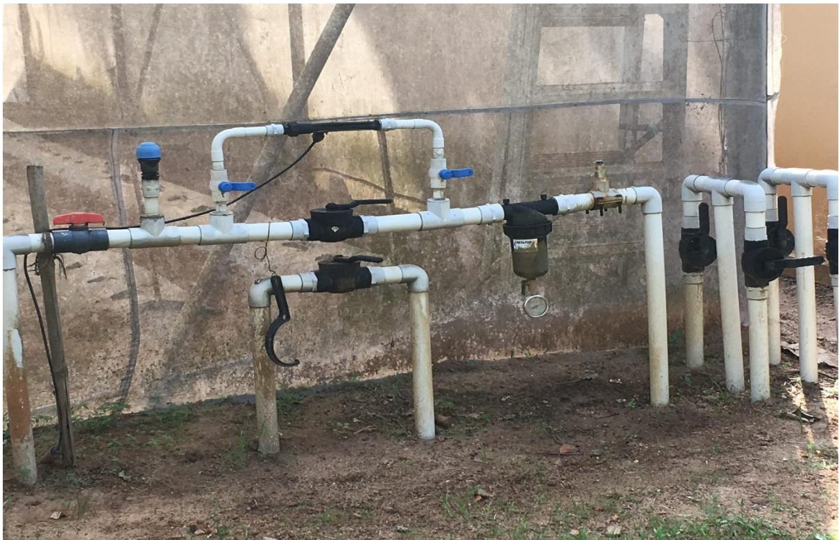
Drip and fertigation system installed in polyhouse
