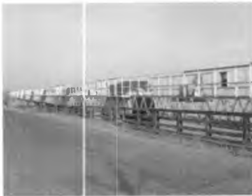
Figure 3.12 Thanneermukham Barrier for preventing salinity intrusion.
