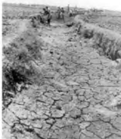
Figure 3.15 A typical field drain used for surface drainage
