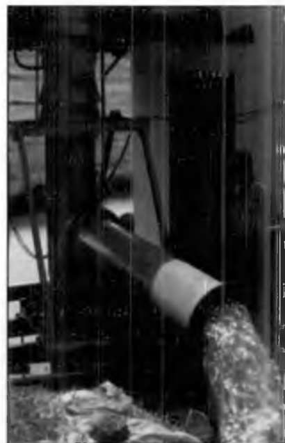
Plate 1.4 Vertical axial flow pump installed at Kole lands of Karalam, Thrissur
