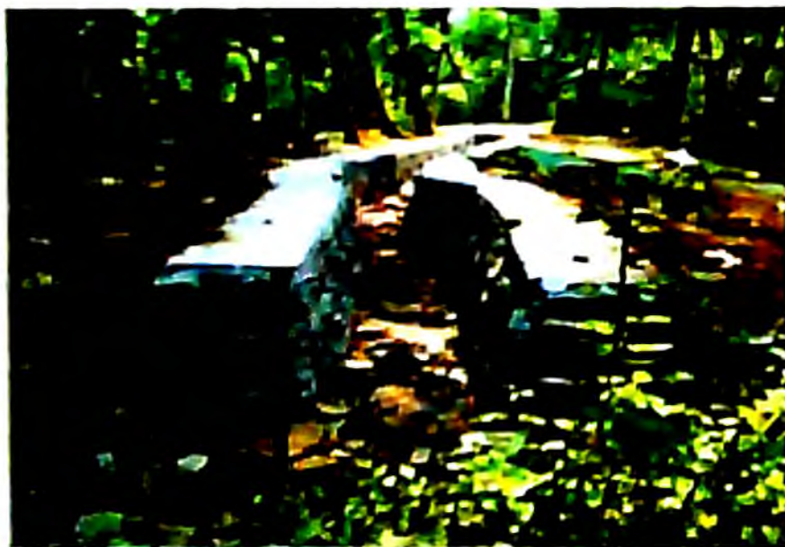
Encroachment of water channels with private walls
