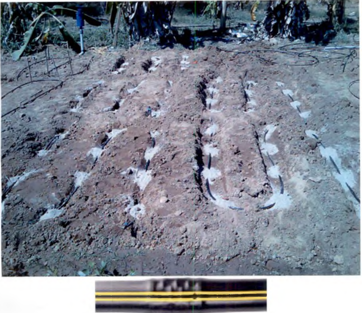
Plate 2. A view of subsurface inline drip and its installation in the field
