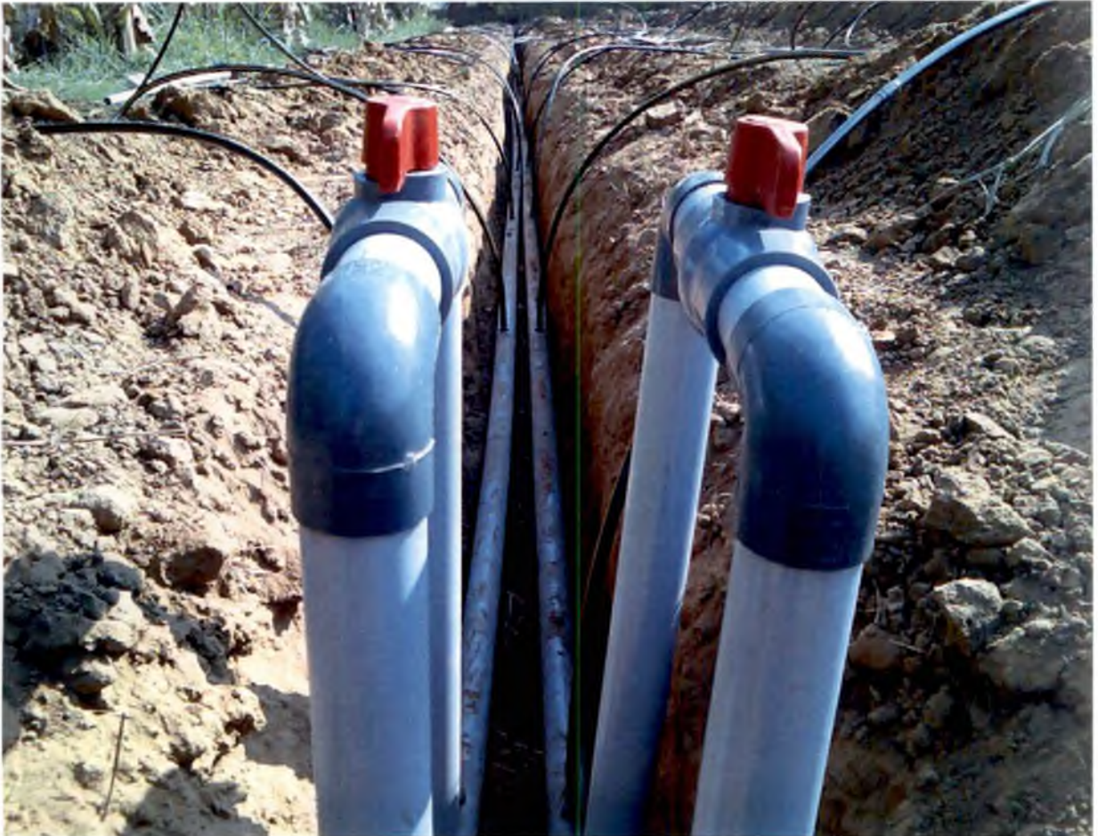
Plate 1. A view of ball valve assembly on sub main to control flow into each block
