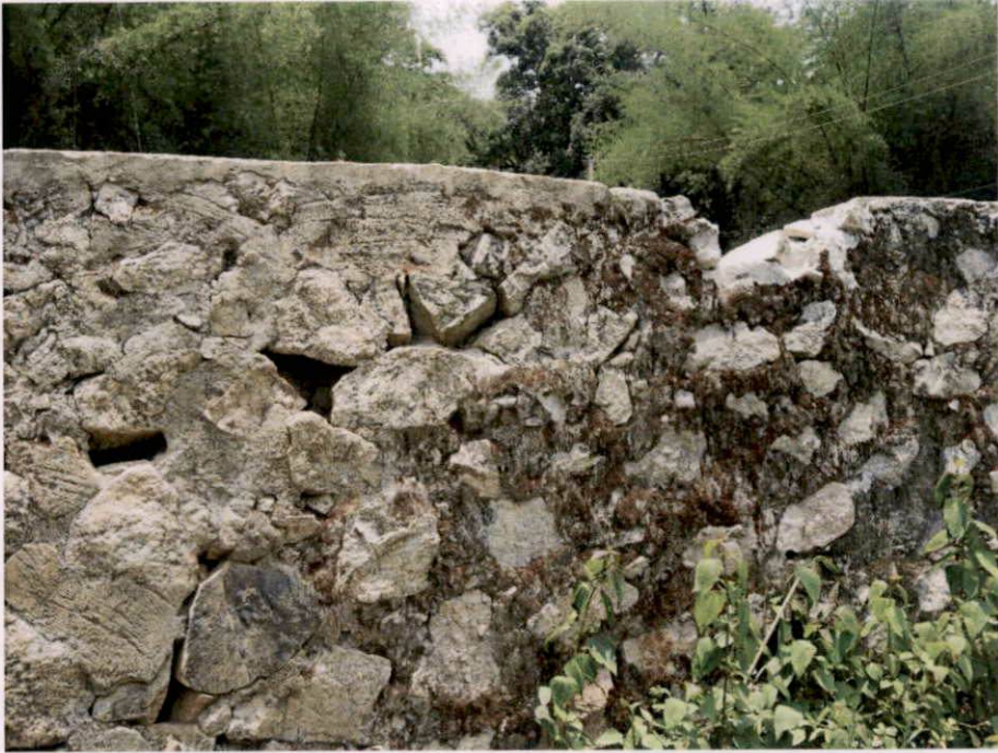
Plate 48. Elephant-proof wall repaired after getting damaged by an elephant at Noolpuzha, Sulthan Bathery
