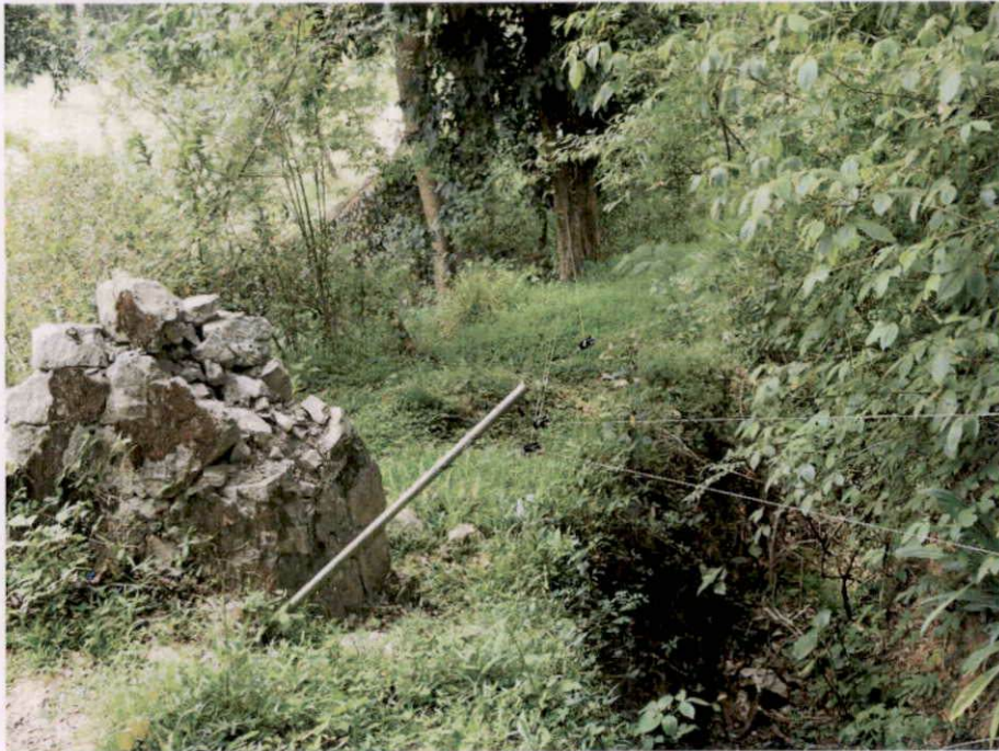
Plate 45. Combination of Electric fence, Elephant-proof trench and Elephant-proof Wall at Noolpuzha, Sulthan Bathery
