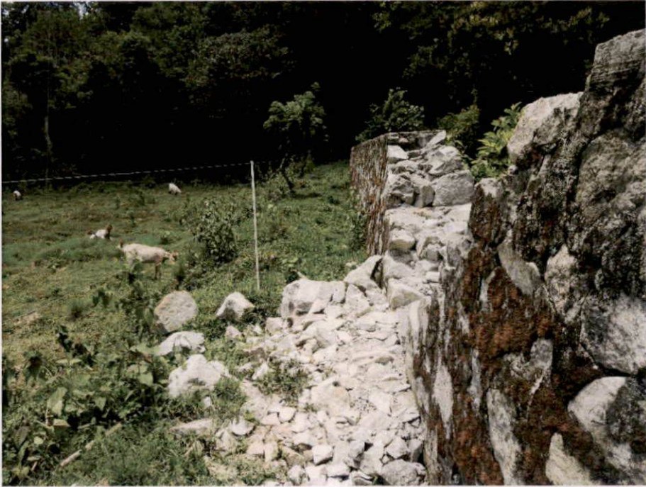
Plate 46. Elephant Proof Wall (with a weak spot) separating forest and agricultural field at Noolpuzha, Sulthan Bathery
