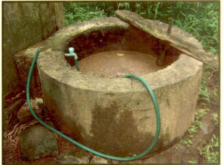
Plate 8. Inlet of biogas unit
