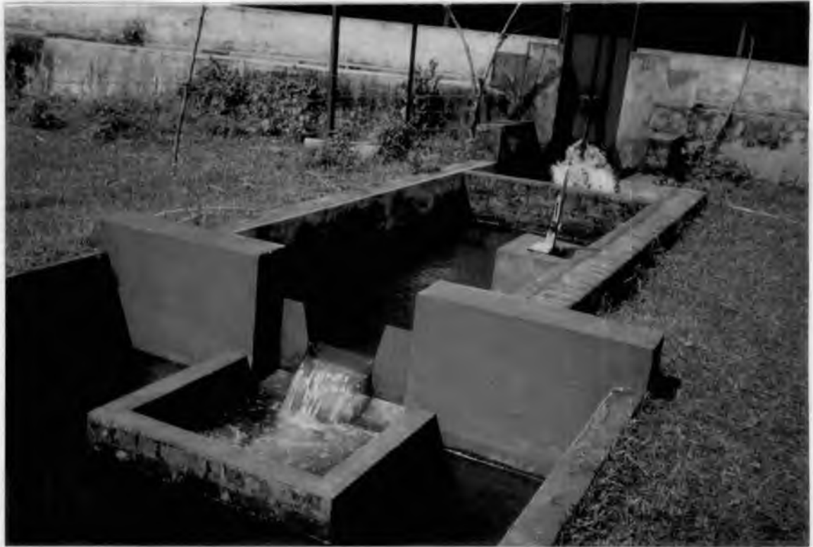
Plate 2 Measurement of flow using Cipolletti weir
