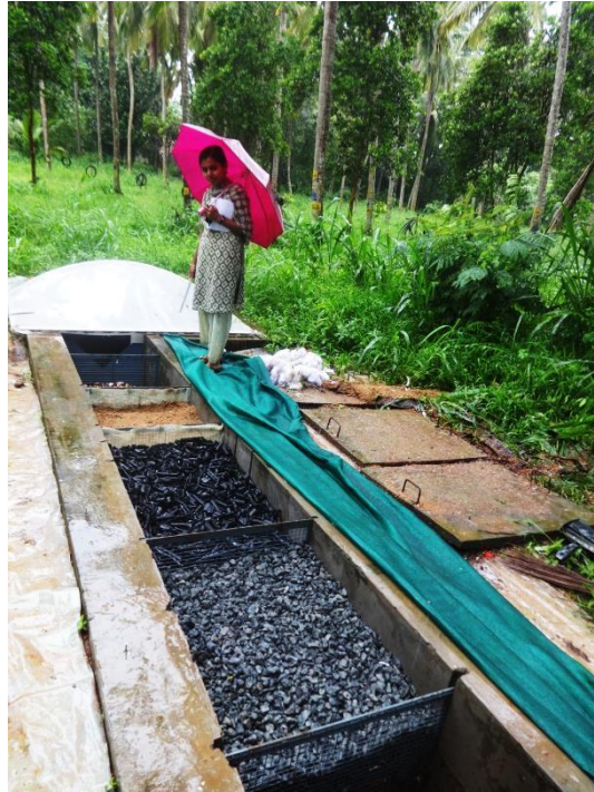
Plate 4.2 View of installed medium combination in the filter unit
