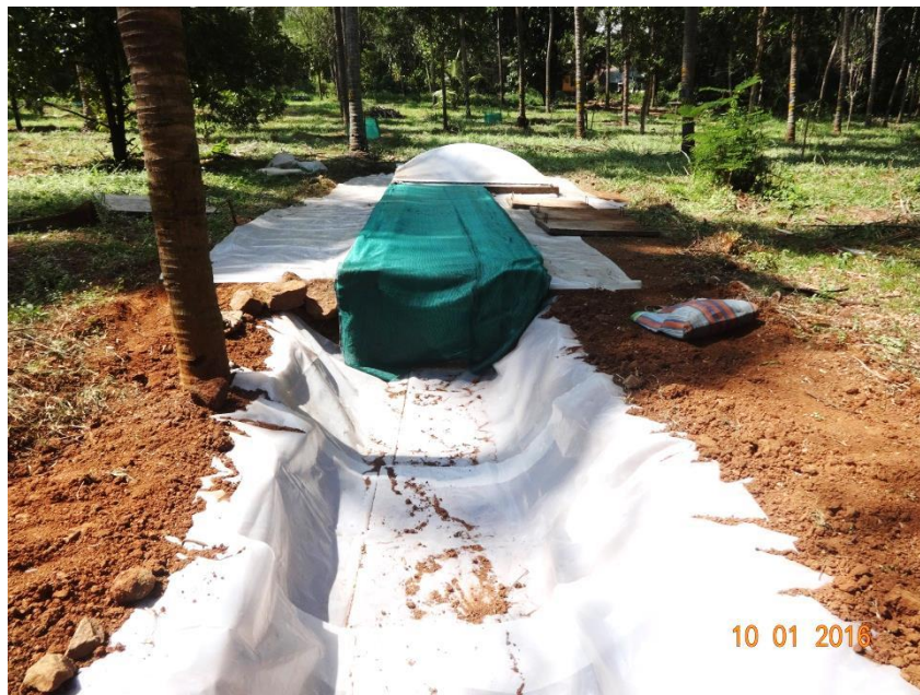
Plate 4.1 Filter unit with conveying channel
